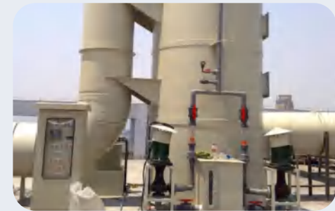
Environmental Protection Equipment
